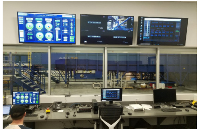
Figure 5: The entire wind tunnel and all of its systems as well as data acquisition are operated remotely from a fully equipped and functional control room.
